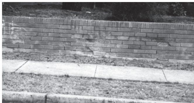
Bricks showing signs of salt and water . Source: DIPNR
